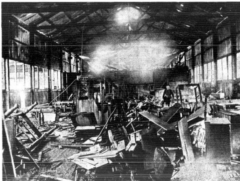
THE APPEARANCE INSIDE THE WORKSHOPS AFTER THE FIRE.
